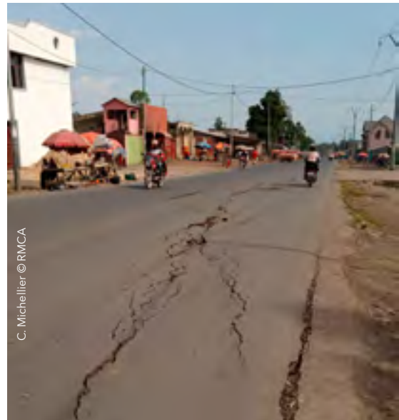
Cracks resulting from the intrusion of the magmatic dyke.
