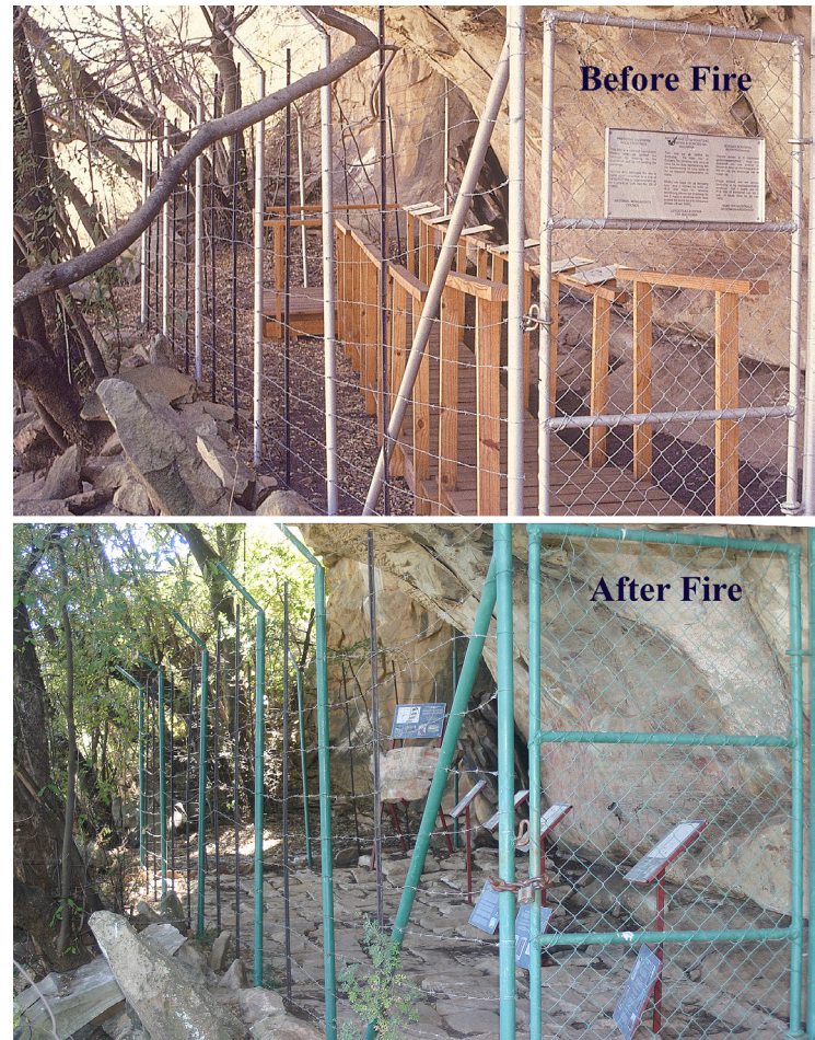
Fig. 1. An example of a wooden boardwalk from a rock painting site in the Free State. The wooden boardwalk and wooden signs burnt in a bush fire, causing considerable damage to the rock paintings. The site was restored using entirely non-flammable materials such as a stone floor and metal signboards. (Upper photo © G. Blundell; lower photo © B. Smith.)
